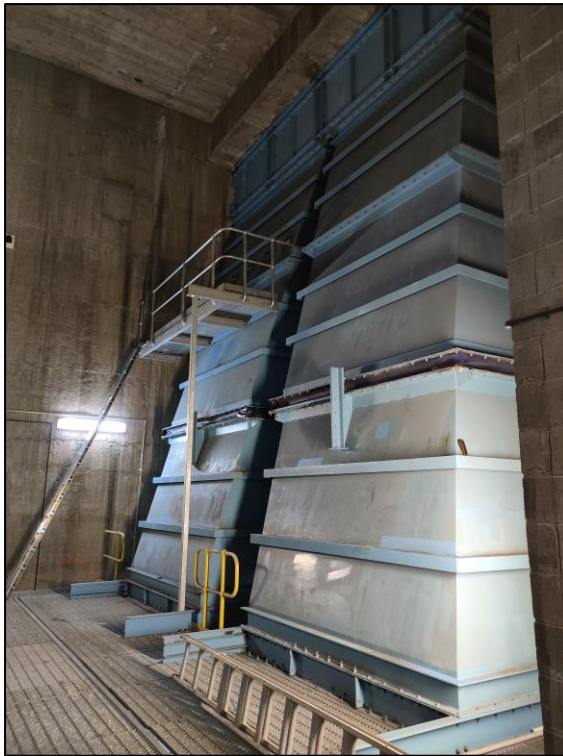
Inside ventilation facility
